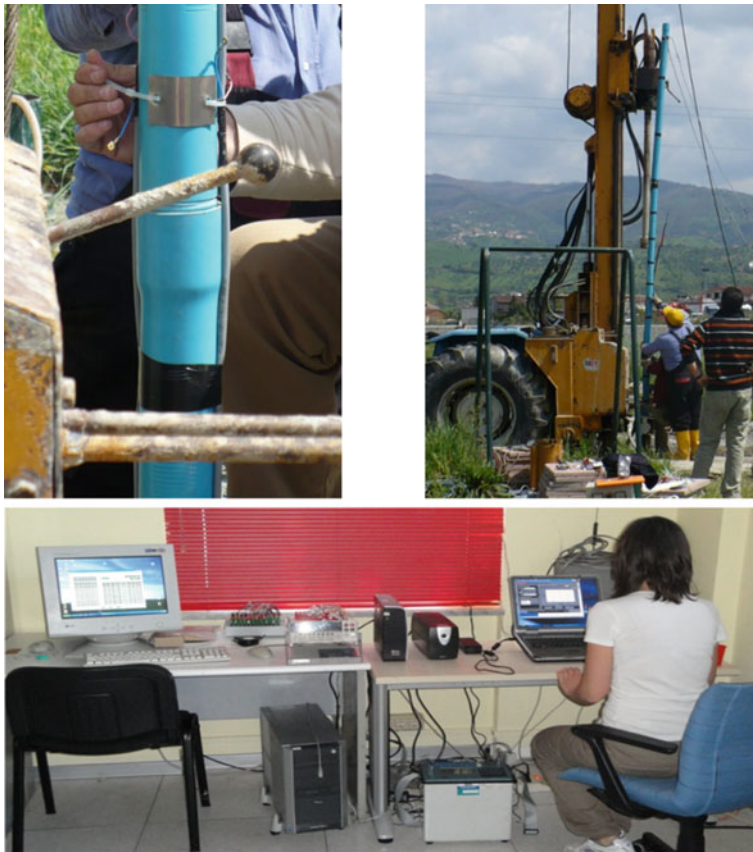
Fig. 16.5 Phases of installation of borehole electrodes for geoelectrical measurements at test site
