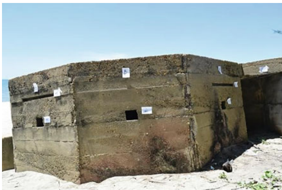
Fig. 13 The structure of the British pillbox in Kg. Pantai Chap, Bachok Source Field study
