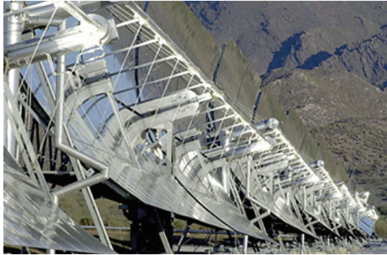
Fig. 3. PTC Kramer Junction (California, USA) [6]
