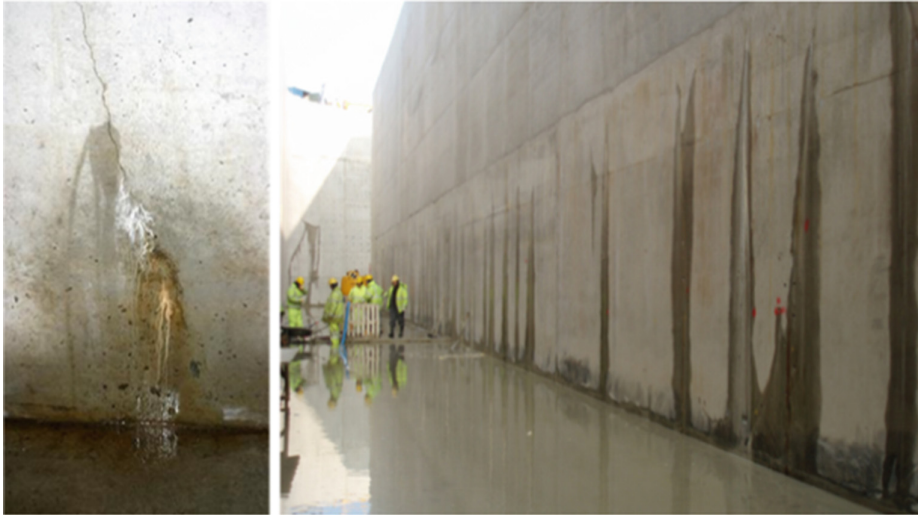
Fig. 1. Water leakage through vertical early age cracks in a wall-slab connection.
