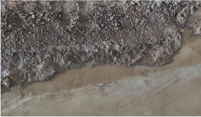
Fig. 21.4 Soil erosion at the entrance of the test section
