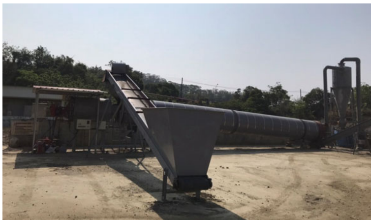
Fig. 31.6 The treatment system of real field thermal desorption
