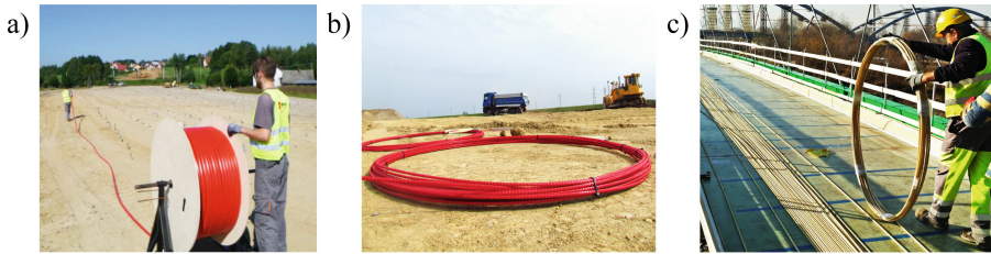
Fig. 3. Sensors delivery to site: a) on a drum [11]; b) c) in coils cut at desired lengths [8].
