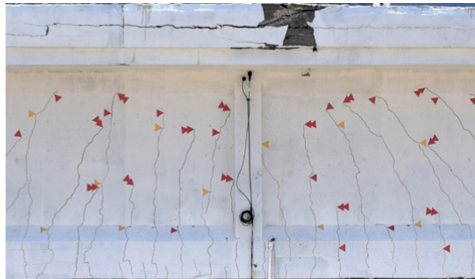
Fig. 6. Visible cracks in the middle of the girder T4 opened during the loading phases P3 (amber triangles), P4 (single red triangles), and P5 (double red triangles).
