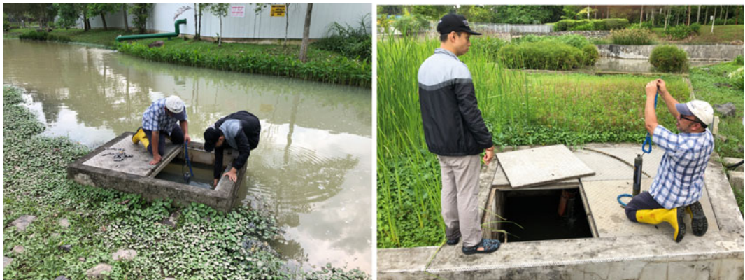
Fig. 6.7 Installation of datasondes at an intake sump upstream of the cleansing biotope in Jurong Ecogarden, Singapore (left), and in the effluent sump from the cleansing biotope, with the biotope cells in the background (right) (photos by the authors)
