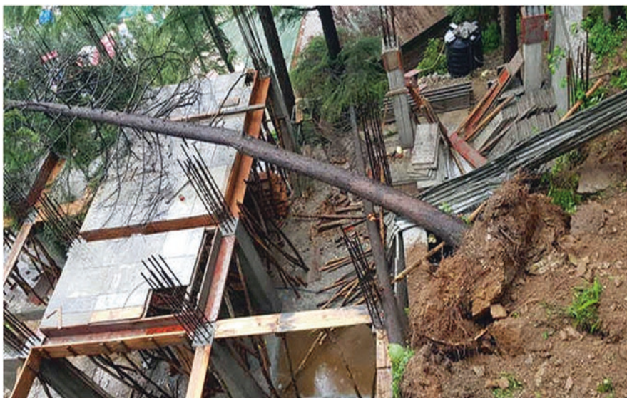
Fig 15.5 Image showing over-excavation of sloppy debris which led to the fall of trees
