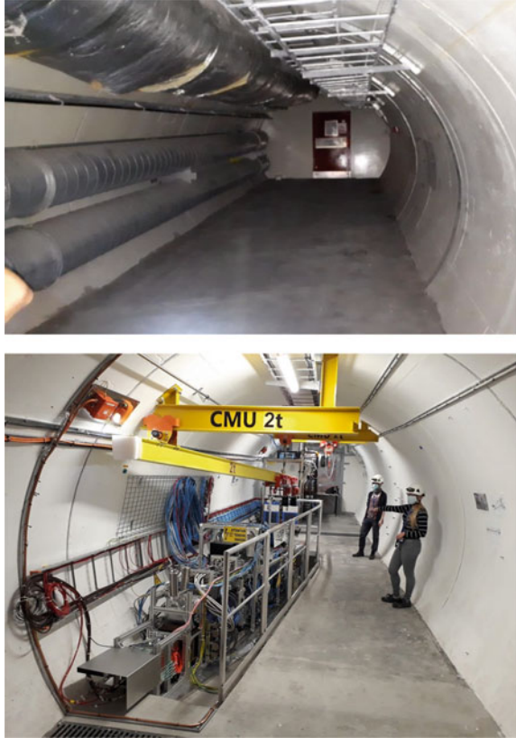
Fig. 4 Top: The TI12 tunnel in December 2019 before civil engineering works and detector installation. Bottom: The FASER detector after installation in the TI12 tunnel in April 2021
