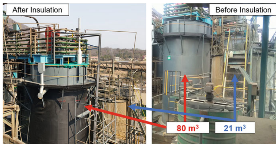
Fig. 4.3 Views of the engineering ( 21 \text{ m}^3 ) and demonstration ( 80 \text{ m}^3 ) scale thermophile reactors
