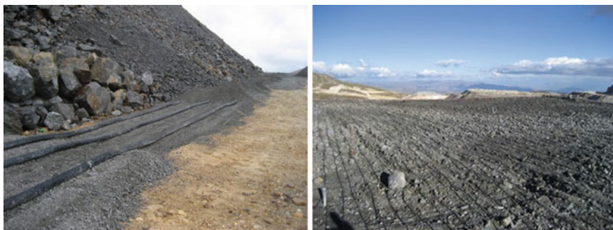
Fig. 10.2 Air distribution pipe at the base of a crushed ore cell during installation (left) and the drip emitter array at Yanacocha (right)
