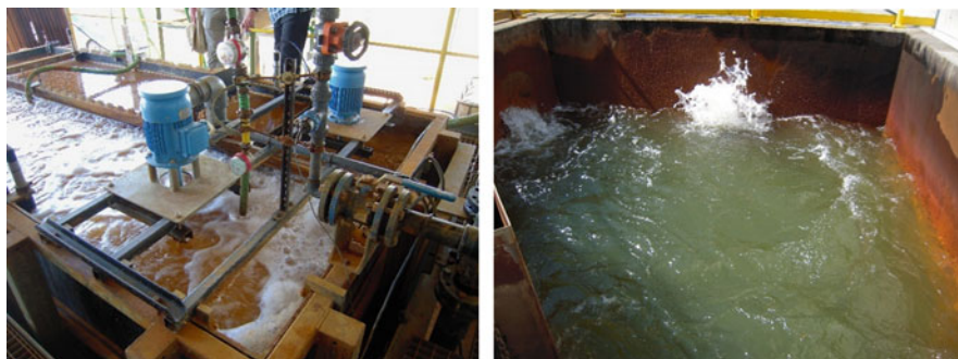
Fig. 16.2 (a) Microbial iron oxidation and precipitation plant treating mine waters from a lignite mine in Nochten (Germany) (left picture). (b) Aeration tank of the plant with untreated mine water (right picture). (images provided by D.B. Johnson)
