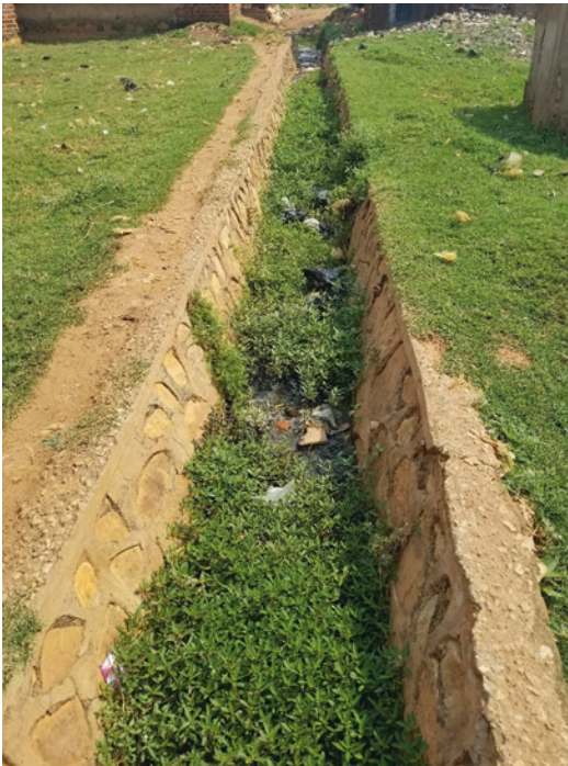
Fig. 18.8 Some drainage canals like this one in Kalerwe are fully covered by vegetation
