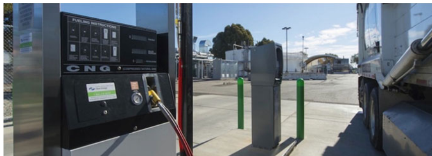
Fig. 20 Refueling station at the site (image courtesy of Cleanworld)
