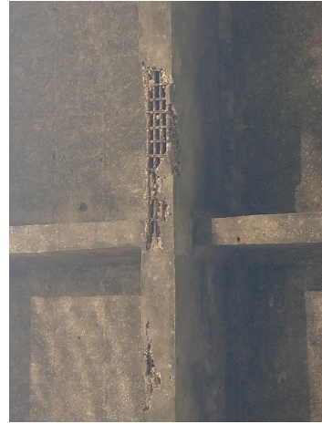
Fig. 5. Damage to girder on deck 6.
