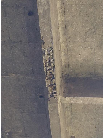
Fig. 4. Damage to girder on deck 4.
