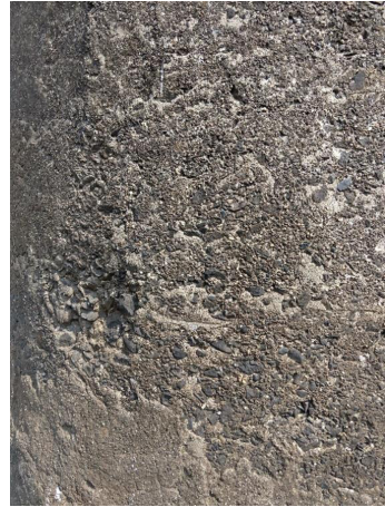
Fig. 3. Surface damage on the piers.
