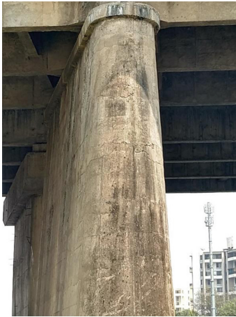
Fig. 2. Horizontal and vertical cracks in the piers.
