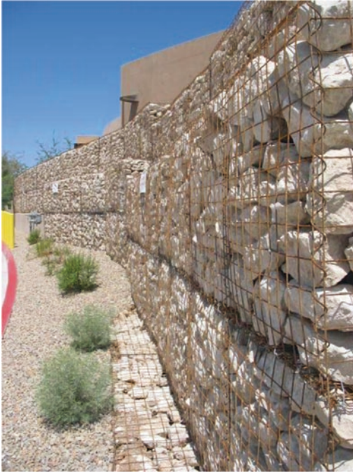
Gabion walls assembled with local stones provide screening of work areas. (Credit for Las Vegas Springs Preserve Photos: David Thaddeus)
