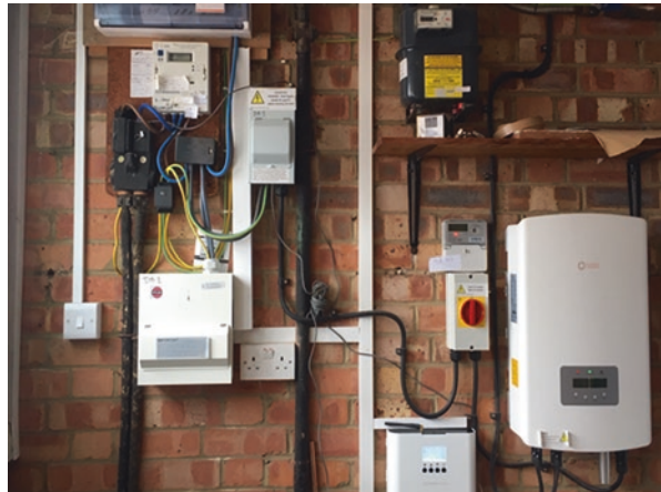
Fig. 2 Distribution boards and control
