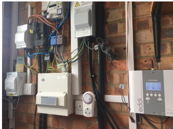
Fig. 4 Lower distribution board (EDDI (DWH diverter) (lower right)
