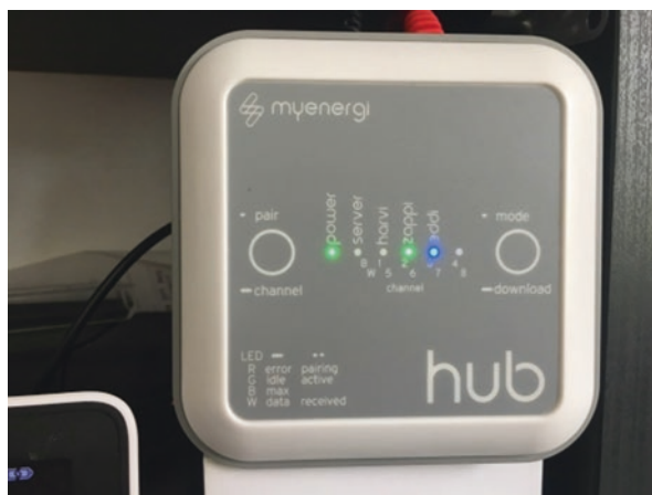
Fig. 5 Blue light shows tank up to temperature (60 C)
