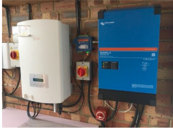
Fig. 13 Two inverters: On the left, the PV inverter; on the right, a charge inverter which controls the 10 kW battery system
