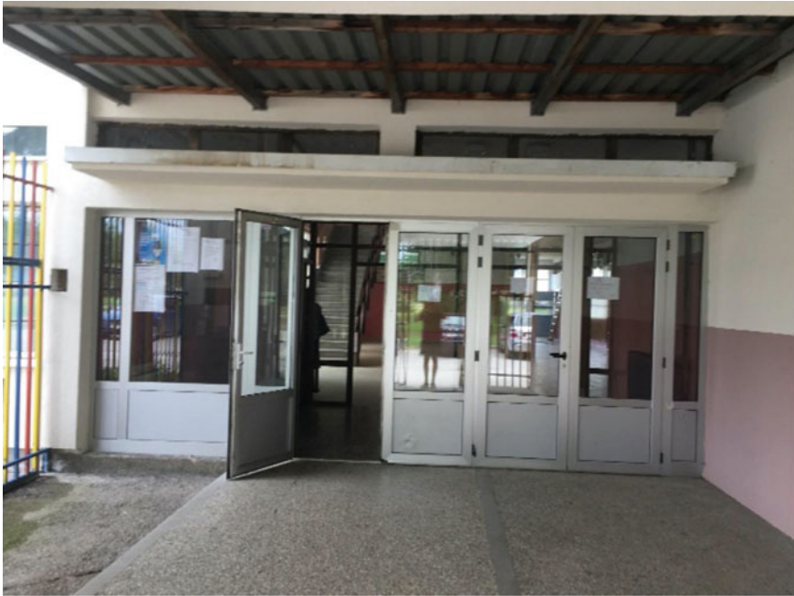
Fig. 10.2 TSUOR in Bosnia and Herzegovina: Two Entrances to a TSUOR School (author's photo, June 2019)
