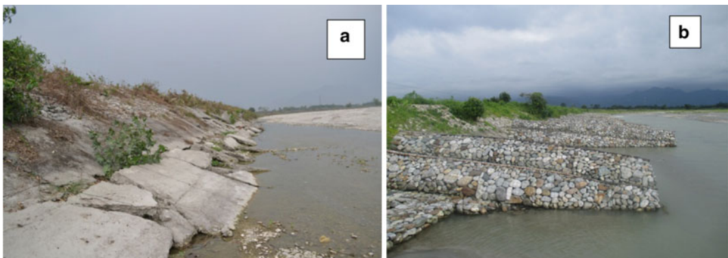
Fig. 2.19 Damaged right embankment at transverse section C–D (a) (photograph was taken on 21.03.2013). Repairing and strengthening of the embankment by addition of dykes (b) (photograph 10.08.2014)
