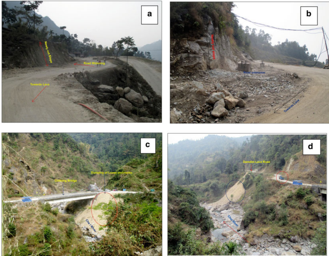
Fig. 2.24 Road widening at near Ambik T.G. (a); road widening near Chittong Bridge (b); dumping of loose sediments generated during road widening into the
