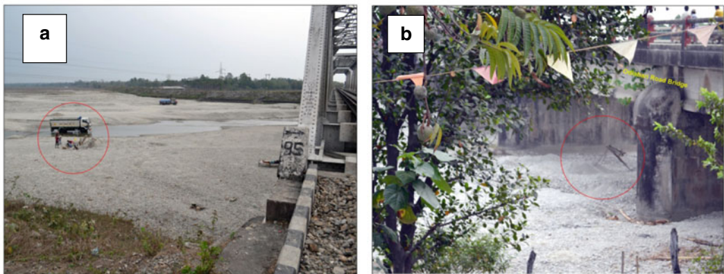
Fig. 2.11 Sediment mining operating barely 100 m upstream of the Odlabari rail bridge (a); sediment mining operating under the Odlabari Road Bridge (b). Photographs were taken on 21.03.2013
