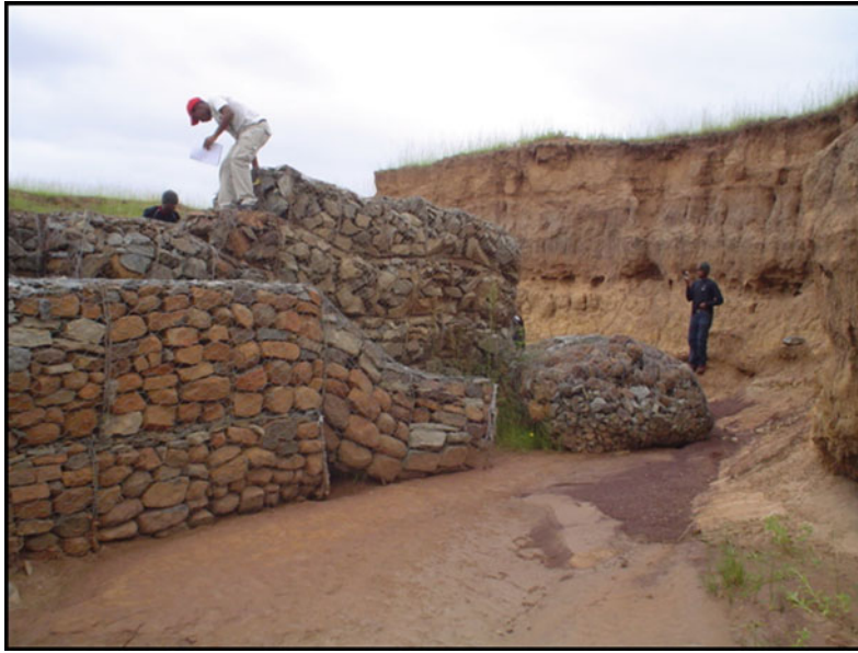
Fig. 11.21 A failed gabion structure in a gully eroded into a dispersive soil in the Eastern Cape Province, South Africa
