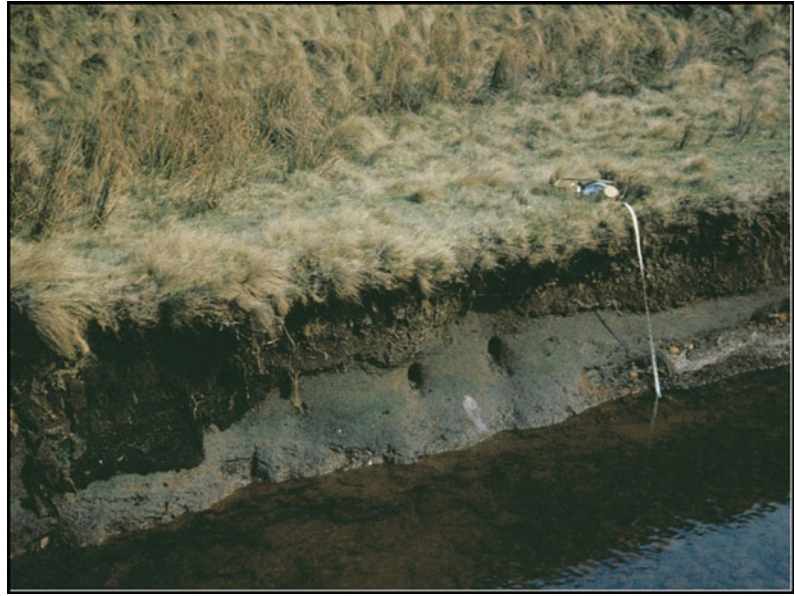
Fig. 11.1 Bank pipes on Burbage Brook, Derbyshire, showing signs of leakage, as seen by a lunchtime observer in 1968
