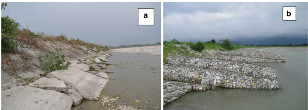
Fig. 2.19 Damaged right embankment at transverse section C–D (a) (photograph was taken on 21.03.2013). Repairing and strengthening of the embankment by addition of dykes (b) (photograph 10.08.2014)
