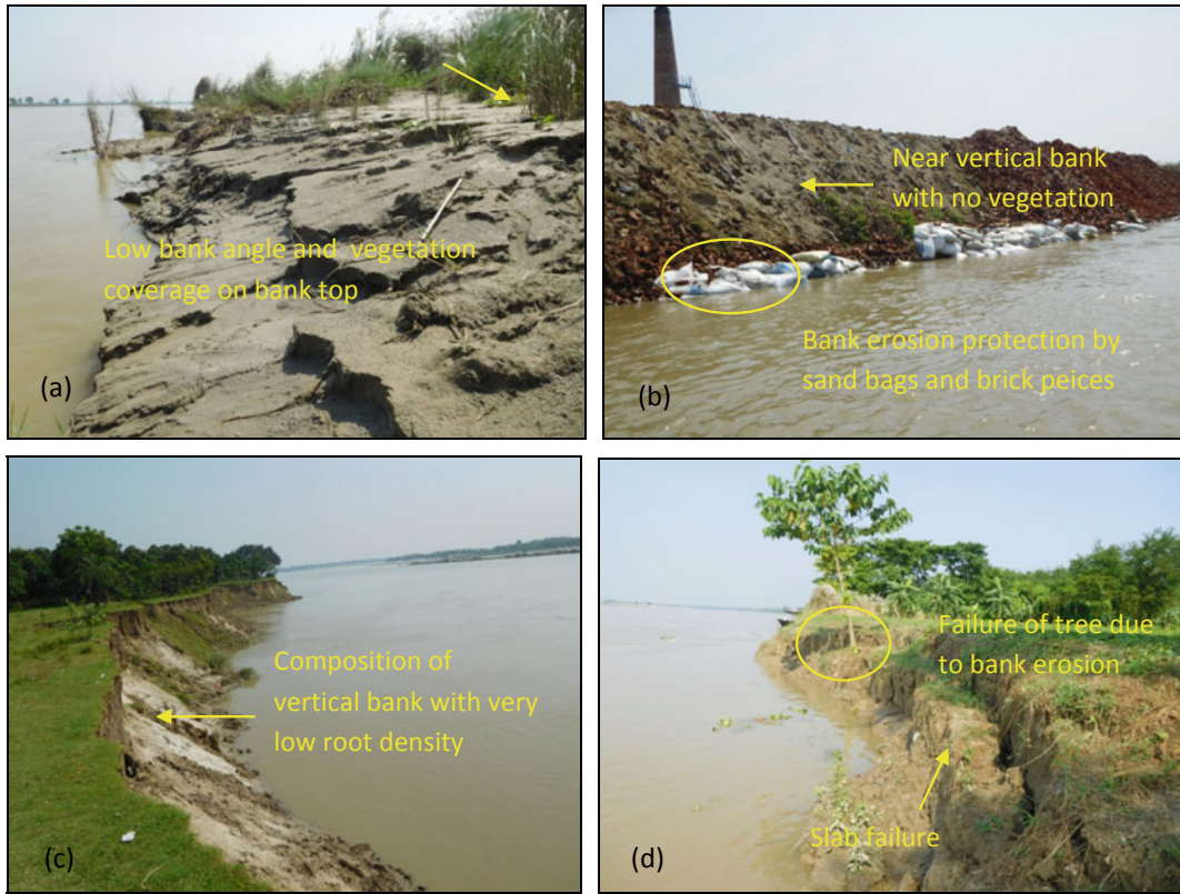
Fig. 6.8 Conditions of river banks. a Right bank at Krisnadebpur. b Right bank at Guptipara brickfield. c Left bank at Santipur. d Left bank between Par Niamatpur and Balagari Char
