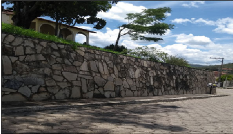
Fig. 6.8 Retaining wall built with stones in the town center. (Source: Pimentel, 2019, p. 68)
