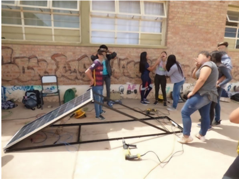
Fig. 11.2 Photovoltaic supporting structure. (Source: Authors' own work)
