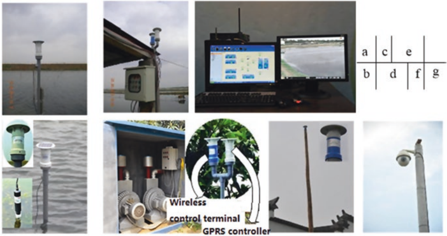
Fig. 2.12 Physical diagram of the wireless oxygenation control system. (a) Water quality monitoring point 1, (b) Water quality monitoring point 2, (c) Water quality control point 1, (d) Water quality control point 2, (e) Site monitoring center, (f) Relay node, (g) Video monitoring equipment
