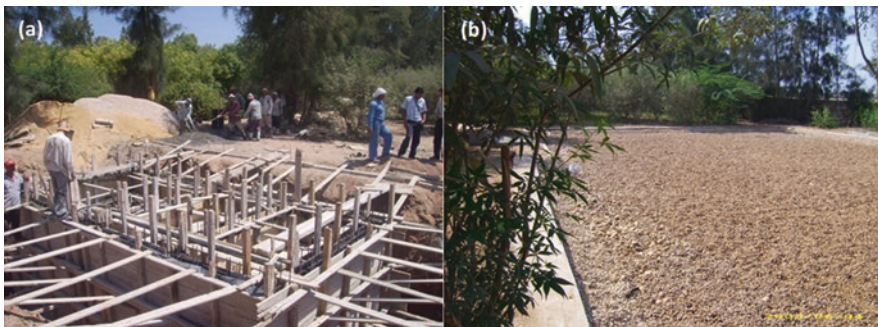
Fig. 5.8 (a) Construction of the septic tank, (b) Constructed wetlands before planting in Sharquiya
