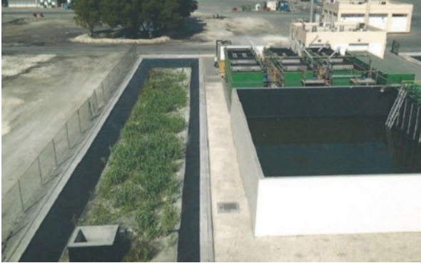
Fig. 15.6 The first STW system in Bahrain (Source: Blumberg Engineers)
