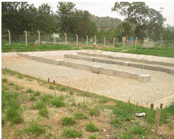
Fig. 9.3 Typical baffled HSSF CW in Tanzania. (Photo by J. Katima)
