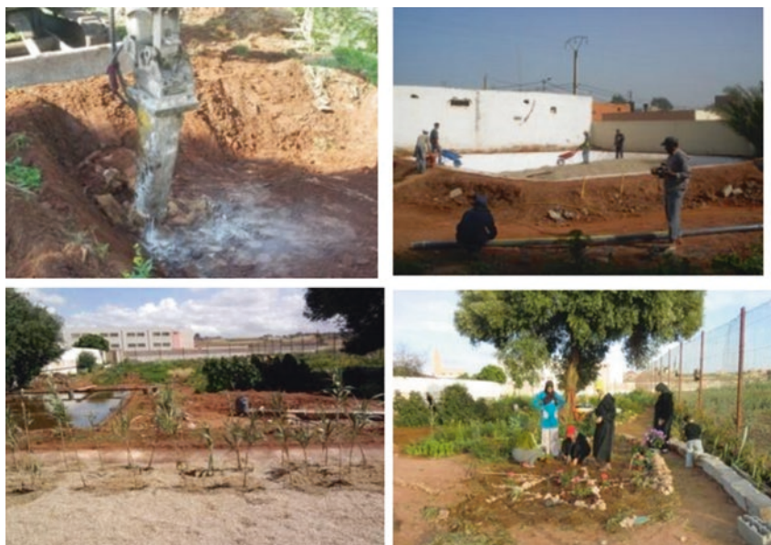
Fig. 6.7 Pictures of the implemented constructed wetland in Casablanca
