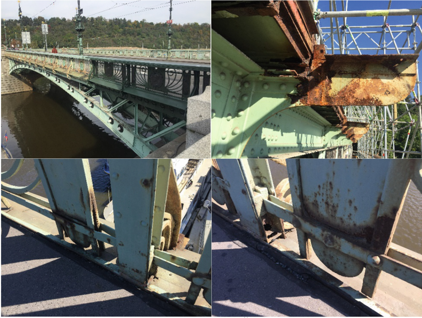
Fig. 2. Current state of corrosion protection of the Čech Bridge railing
