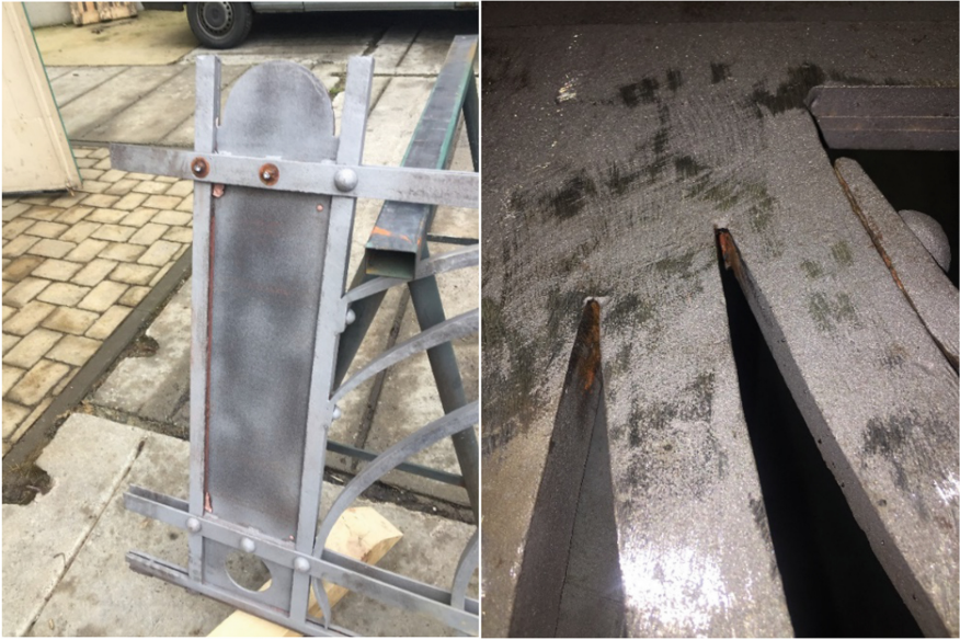
Fig. 4. Pre-treatment of the surface by blasting before application of hot-dip zinc by immersion
