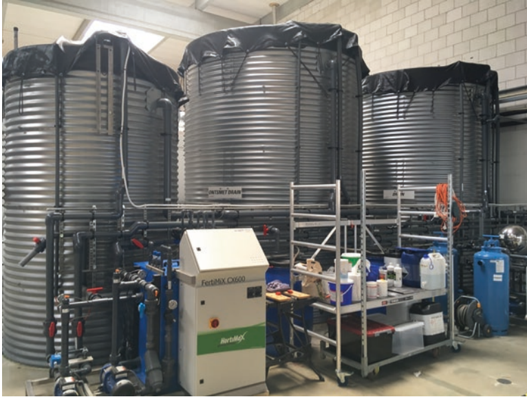
Fig. 6.16 Water tanks and nutrient mixing system
