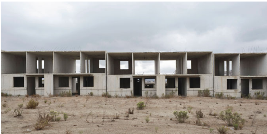
Fig. 19.3 Unfinished low-income housing in Tijuana built by private developers and subsidized by the federal government, 2018. Photo Monica Arreola
