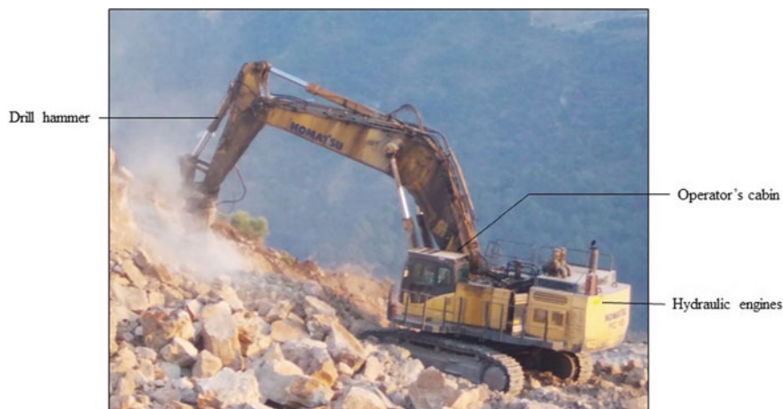
Fig. 10 A rock breaker operating in limestone mine. The dust generated by this process can be clearly seen
