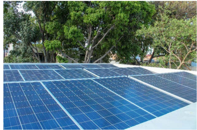
Fig. 2 Shows Photovoltaic station located in roof. (Eosis, 2017)
