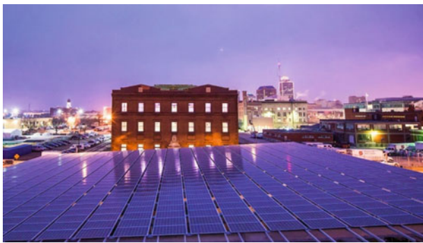
Fig. 4 Shows the photovoltaic panels installed on the car canopy structure. (Bradford et al., 2019)
