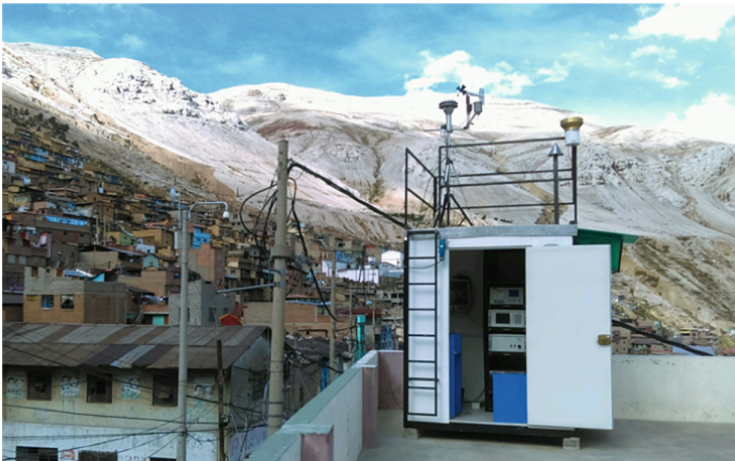
Fig. 2. Environmental station without internet connection.
