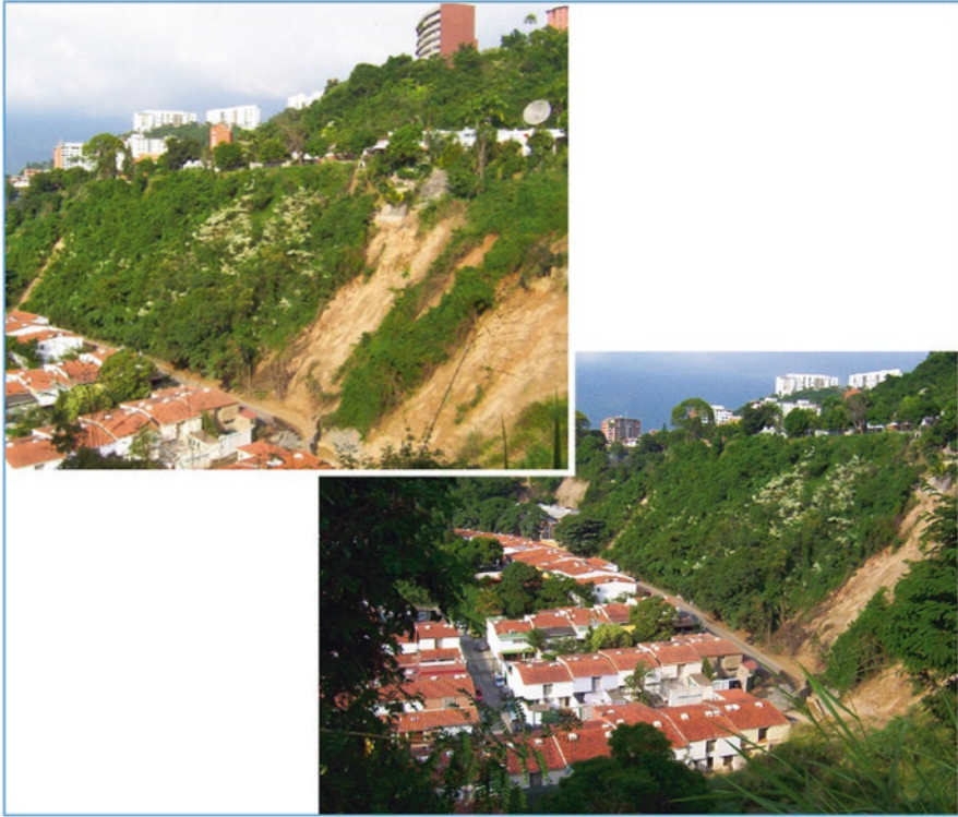
Fig. 12.7 Backfills of excavated material threatening the middle-upper class Santa Inés neighborhood (© J. Rebotier, 2008)
