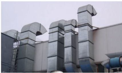
(a) Smoke exhaust duct
