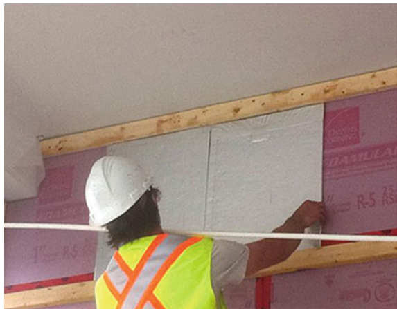
Fig. 10.2 Installation of VIPs for exterior building envelope retrofit in Whitehorse, Yukon, Canada
