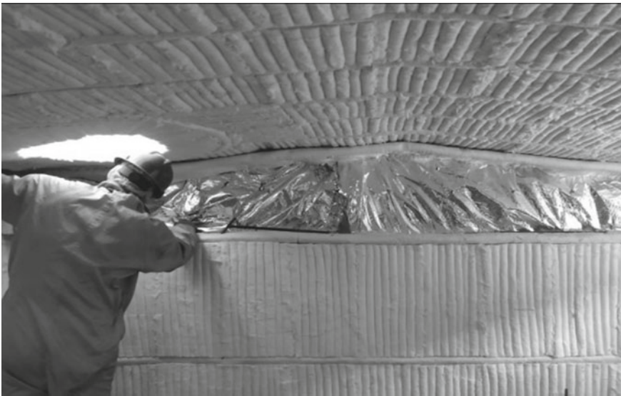
Fig. 5.20 Ceramic wool used in furnace lining
