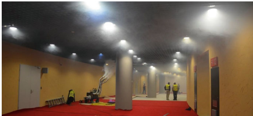
Fig. 11.20 A hot smoke test used in parallel with PDS tests, to determine the system integration and impact of the PDS system on the performance of the smoke control in the fire compartment
