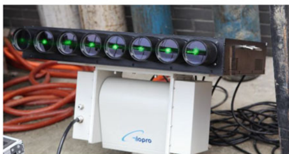
Fig. 13.24 Monitoring column movement with LAMS: (a) Column movement; (b) LAMS system
