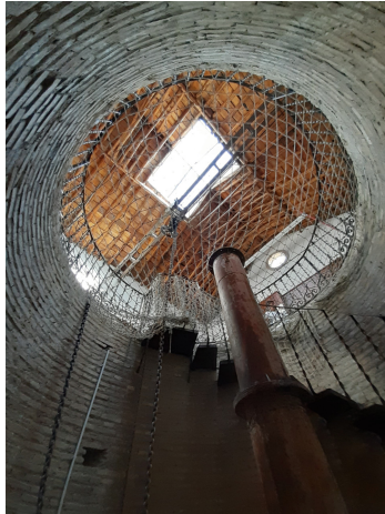
Fig. 8. The access to the well and the helical staircase. From the inside of the well (owner’s collection).
