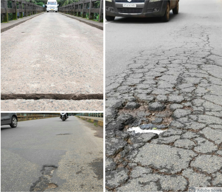
Fig. 1. Bridge deck having irregular road profile.
