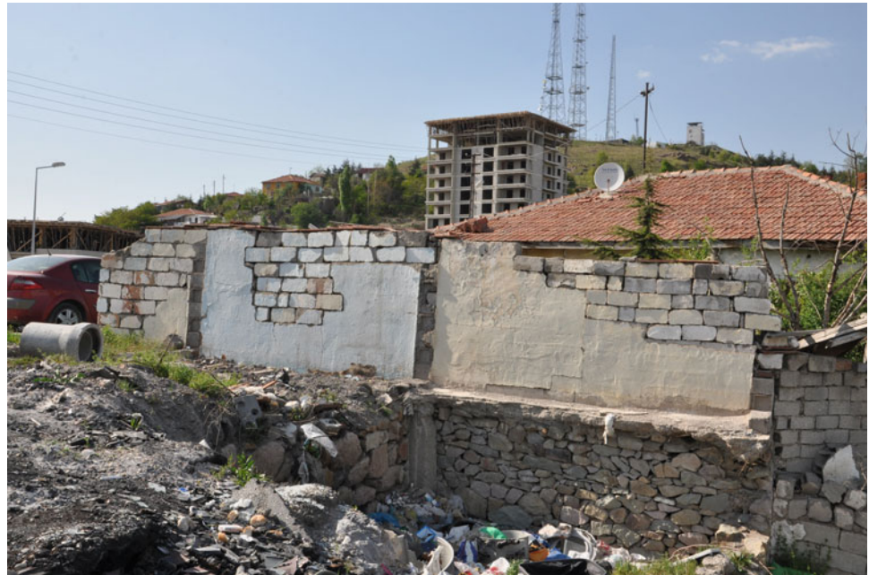
Fig. 24 Material quality of demolished squatter unit. Photograph taken by the author
