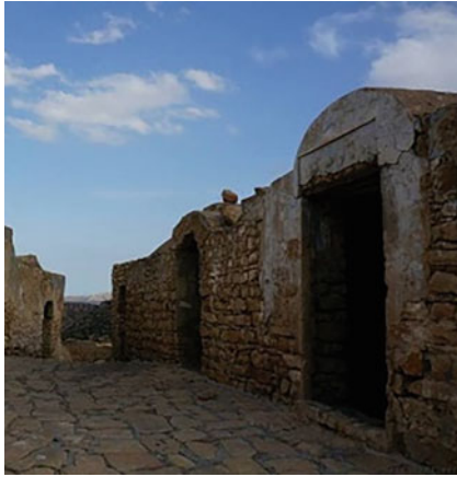
Fig. 15 The house before rehabilitation
