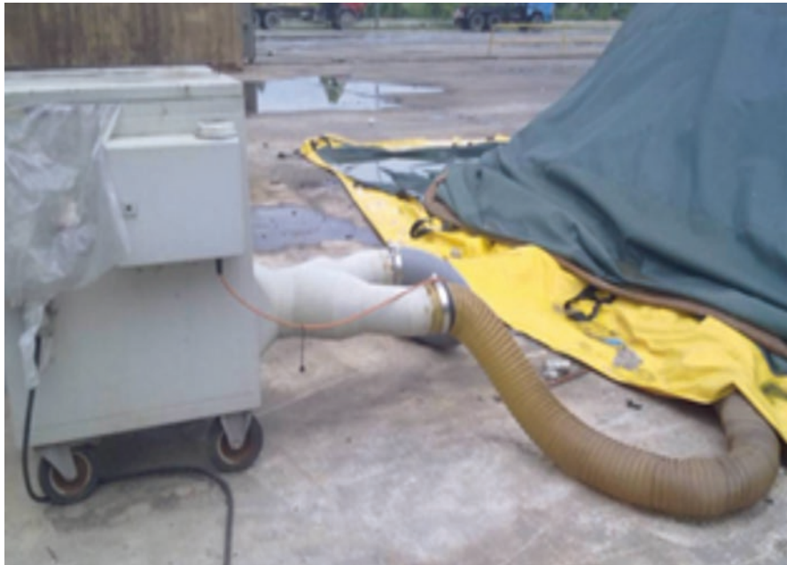
Fig. 7.28 Ventilation pump for the biodrying system
