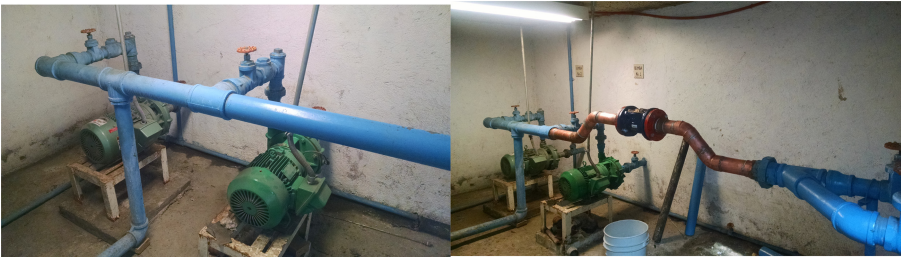
Fig. 8. ESCOM water monitoring system.
