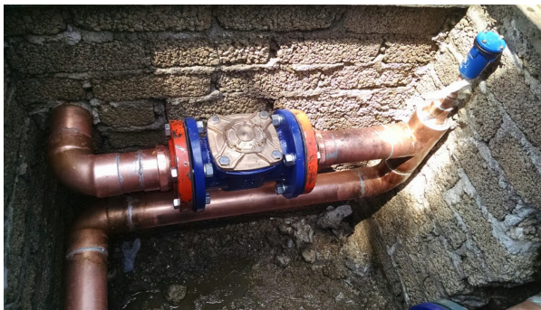
Fig. 6. Water meter installed at CIDETEC.
