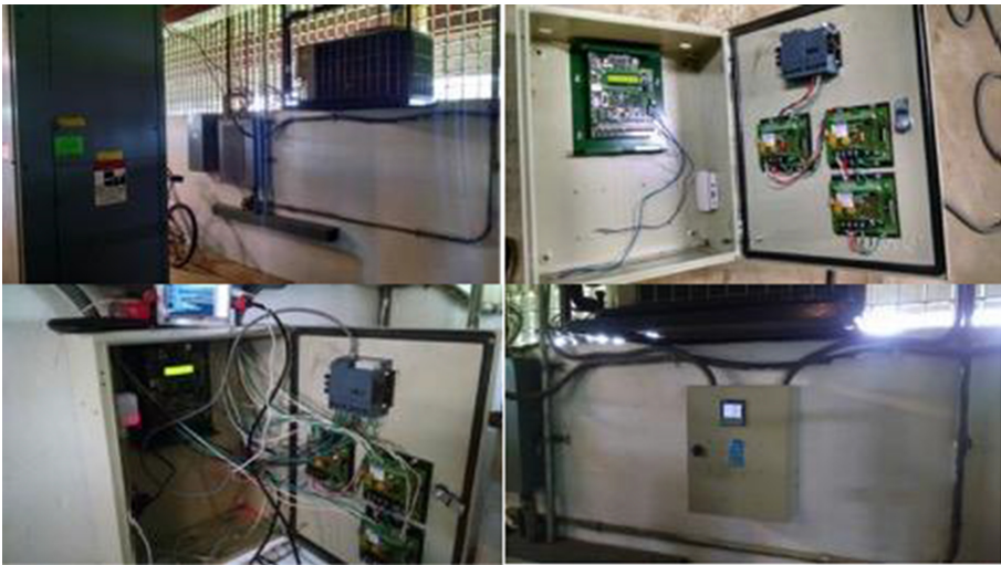
Fig. 3. Meter installation in the CIC substation.
