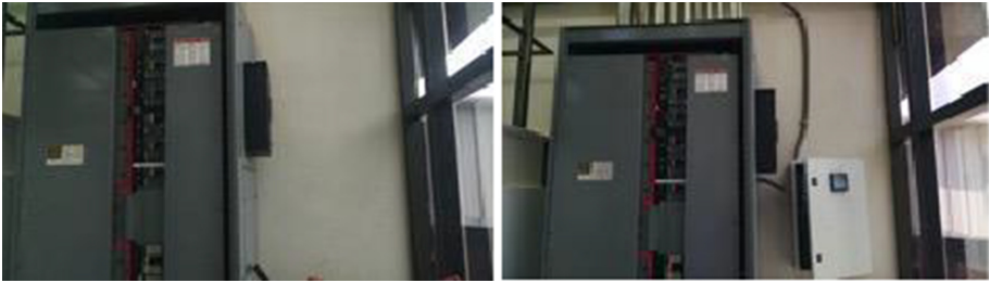
Fig. 5. General dashboard and energy monitoring system at CIDETEC.
