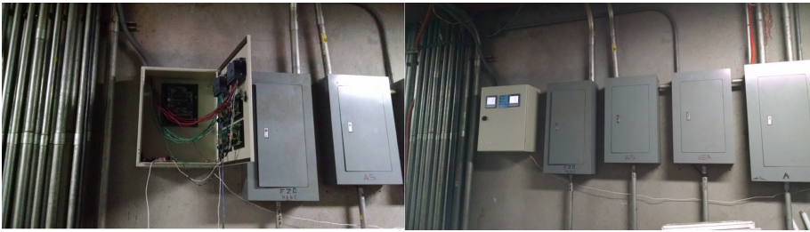
Fig. 7. ESCOM general dashboard and energy monitoring system.
