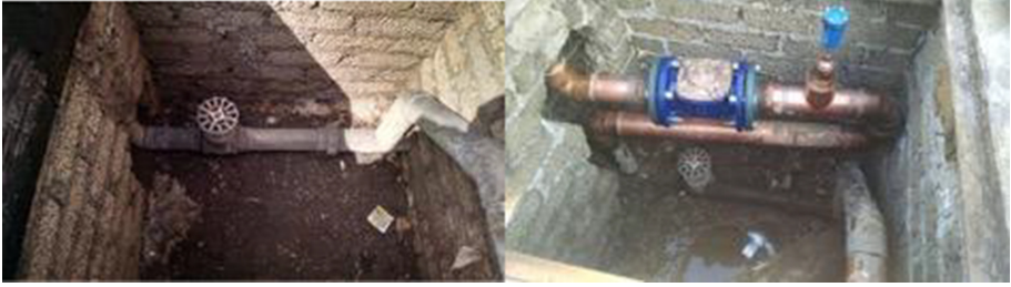
Fig. 4. Water meter installed in the CIC.
