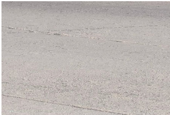
Fig. 5 Transverse cracking in old NH-2
