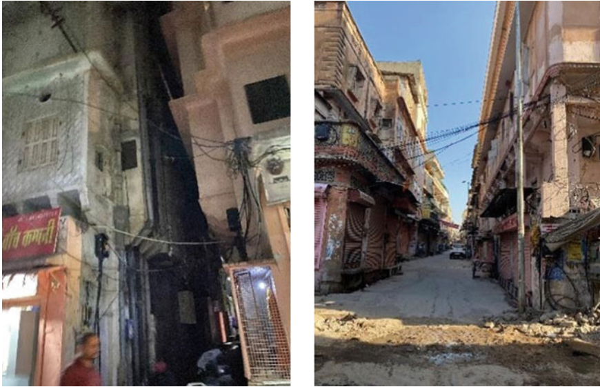
Fig. 5 Images showing the infrastructure facilities being placed haphazardly without considering the heritage character
