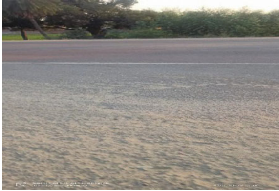
Fig. 4 Block cracking in old NH-2
