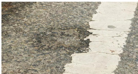
Fig. 10 Slippage cracking in old NH-2
