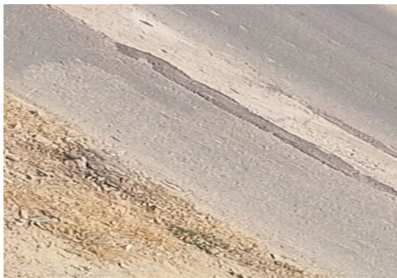
Fig. 11 Rutting at old NH-2
