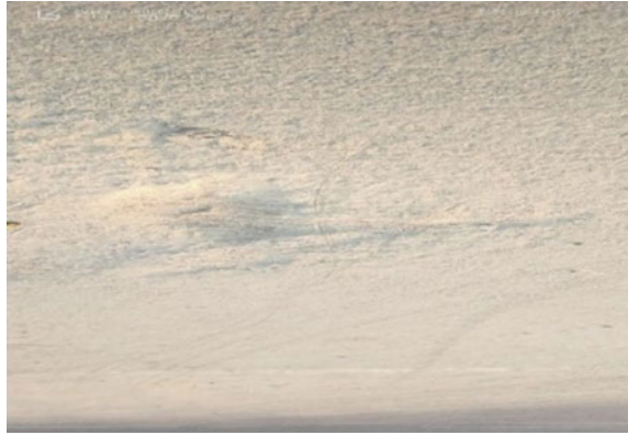
Fig. 6 Pothole in old NH-2
