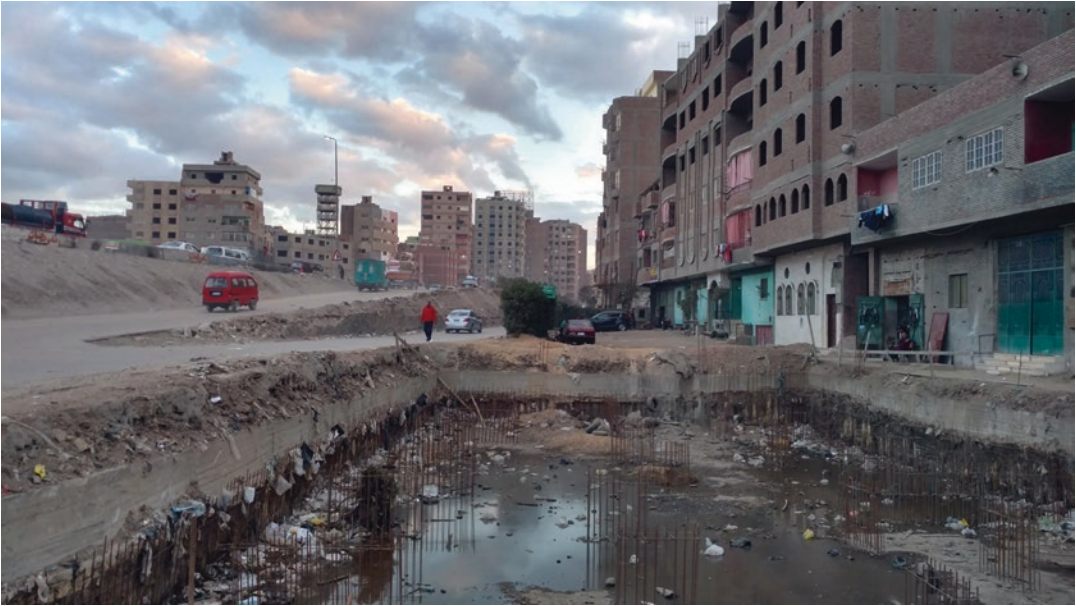
Fig. 4.4 A plot area close to Cairo Ring Road and Ard al-Liwa, being excavated in preparation for construction (CLUSTER 2018)
