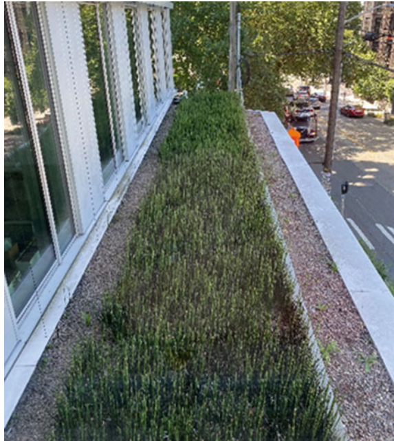
Fig. 8 The 44.6m 2 (480-ft 2 ) graywater treatment wetland is located on a third-floor balcony
