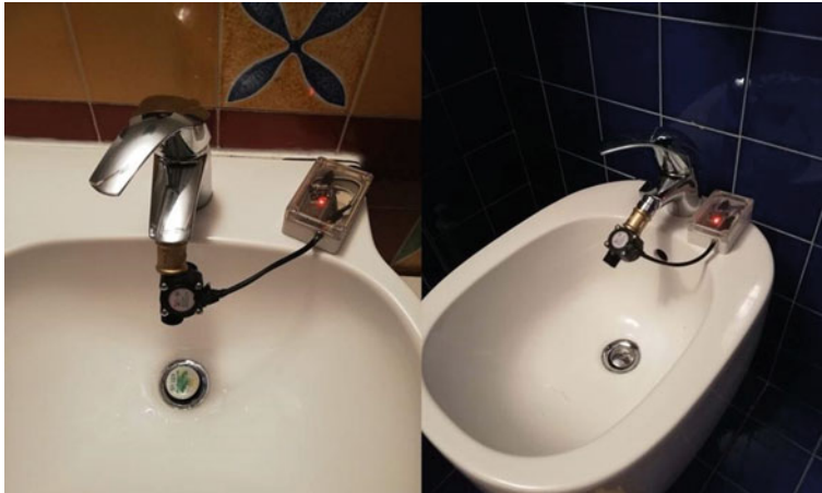
Fig. 5 Shows an example of IoT system installation on water fixtures. Source Authors
