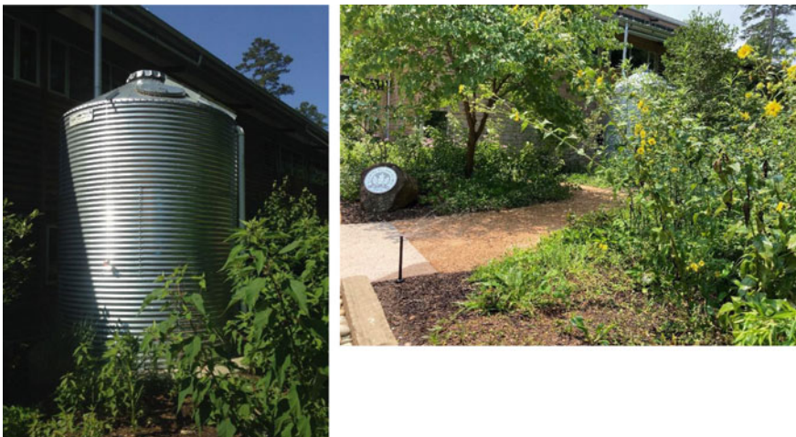
Fig. 3 (Left) One of the seven cisterns used to collect rainwater at the NC Botanical Garden at UNC-Chapel Hill (the one pictured is approximately 18,000 L). (Right) The sprinkler system connected to the RWH system that is used to irrigate the gardens. Photo courtesy of UNC-Chapel Hill
