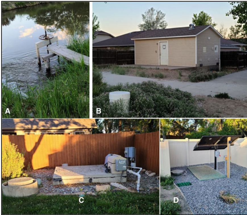
Fig. 13 Types of irrigation pumps used in the Grand Valley. (Photos by author 2021)
