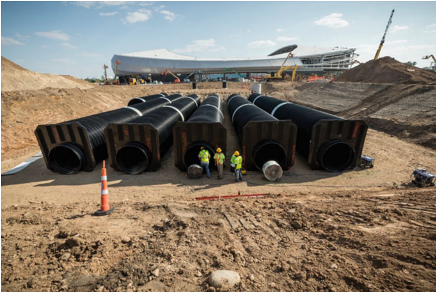
Fig. 8 Installation of underground rainwater storage tank at Allianz Field in St. Paul, MN. Source Public Domain
