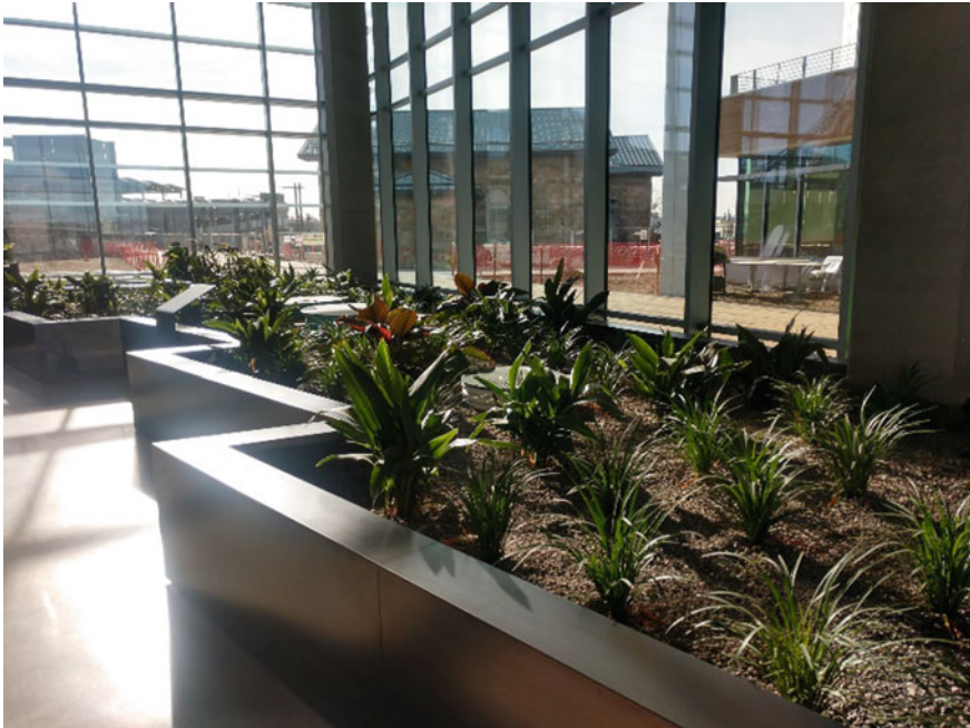
Fig.6 Denver water’s wetland system treating the building’s blackwater in Denver, CO. Source Public Domain
