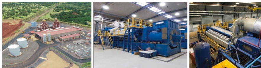
Fig. 10.9 50 MW HECO Schofield Generating Station located on Schofield Barracks, HI
