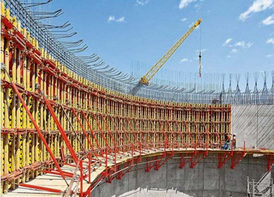
Fig. 7 Typical construction site for retaining wall with reinforcement arrangement and concrete works. (Source: Field Study, 2021)
