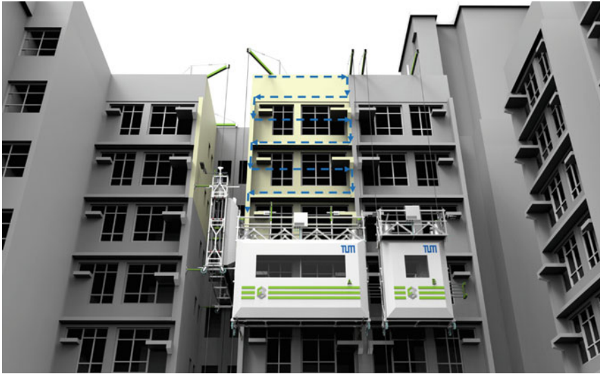
Fig. 4 During the development of the CIC robot, all operations needed from setting up the robot on site, operating it along the façade, to the removal of the robot from the site were carefully planned (source R. Hu)
