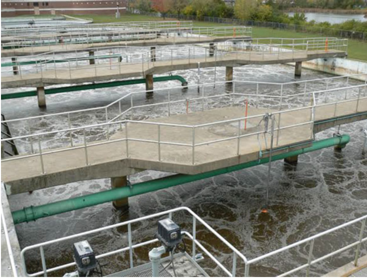
Fig. 5 A photograph of aeration tank [18]
