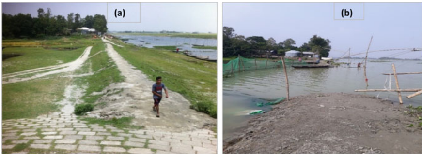
Fig. 3 Breaching location beside Union Parishad from where water enters into the Ranigram area during a dry season and b monsoon
