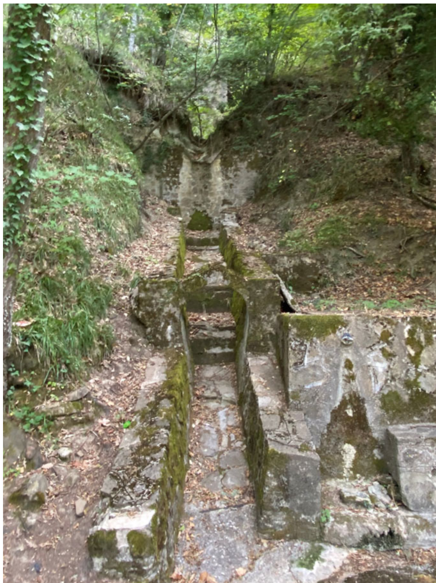
Fig. 51.16 Hydraulic works to reduce water velocity. Source Interregional River Basin Authority of Basilicata
