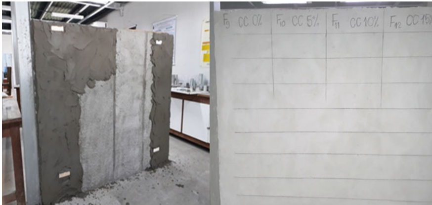
Fig. 8 View of the ceramic block panel during the application of plaster mortar
