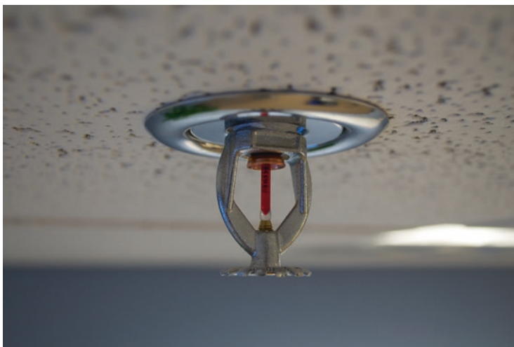
Fig. 10.27 Fire sprinkler ceiling mount side view. (Source: Brandon Leon, licensed with CC BY-SA 2.0)
