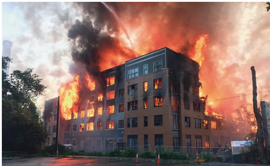
Fig. 10.18 Fire in timber frame apartment building under construction. (Source: Captain John Bonadio, Waltham Fire Department, as published at https://www.enr.com/articles/42484-what-local-officials-want-to-do-about-wood-frame-building-fires-in-massachusetts (last accessed September 2020), Courtesy of Waltham, Massachusetts Fire Department)
