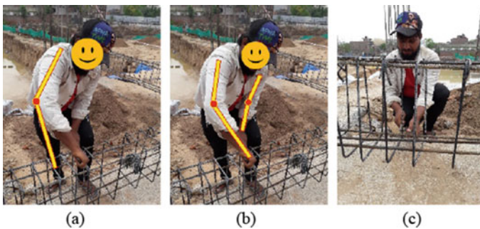
Fig. 3 Worker tying stirrups (back slightly twisted while standing and excessively twisted, knees bent, shoulder stretched while sitting)
