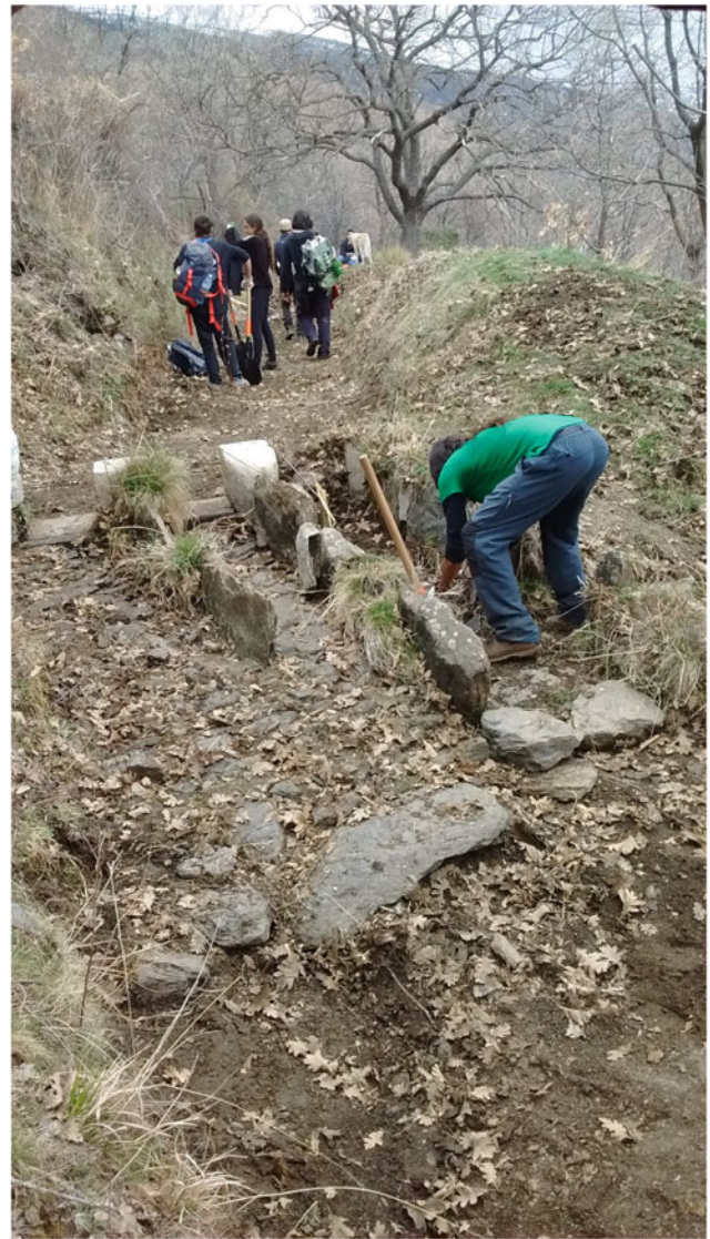
Fig. 5 Group of students helping to clean and repair an acequia de careo (MeMoLa project)
